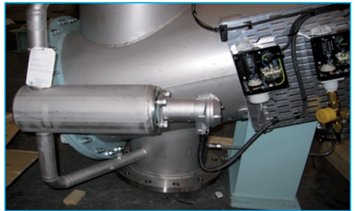
Customized stainless steel float chamber with Trimod Besta level switch for low level alarm.
