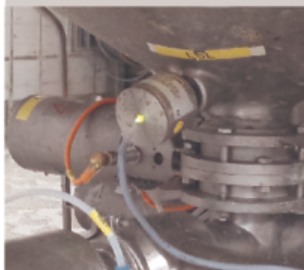
View of installed sensor from the outside
